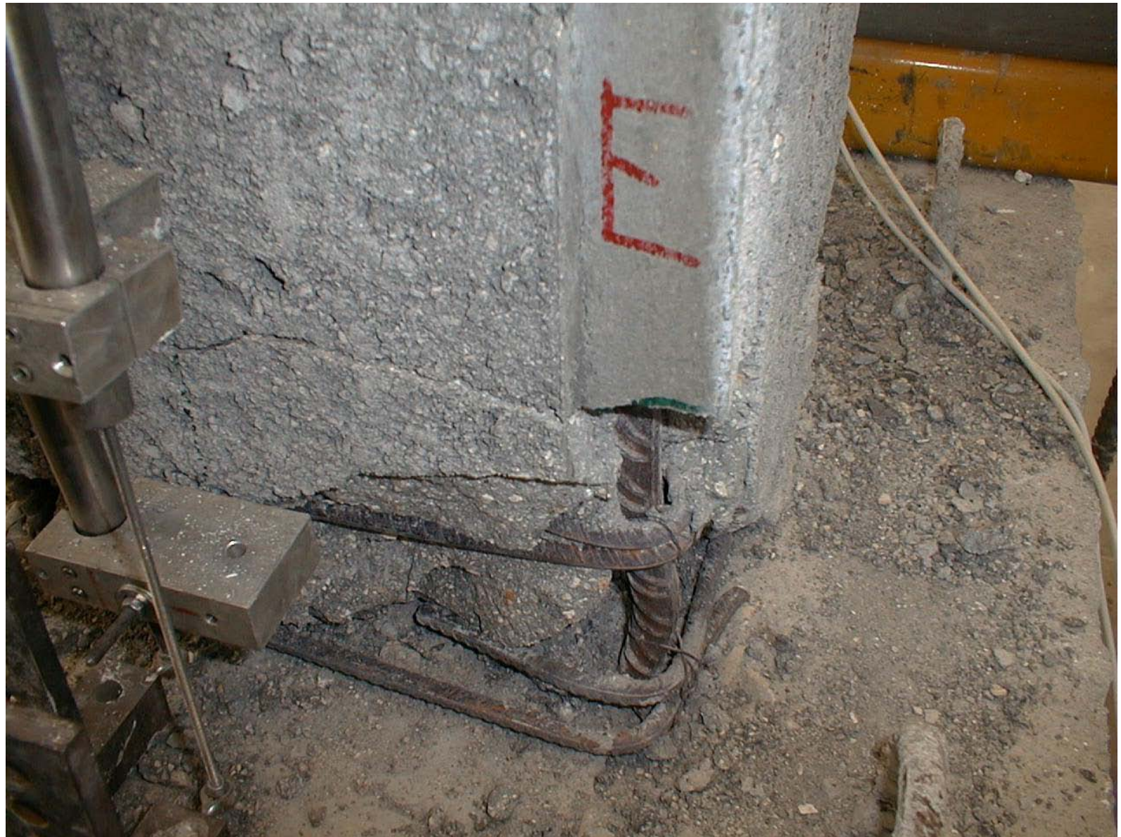
Bar buckling due to stirrup ends opening
